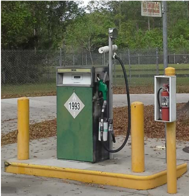
Fuel Pumps Installed in 1986 (33 years ago)
