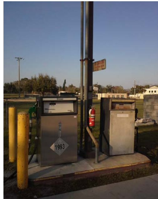
Fuel Pumps Installed in 1991 (28 years ago)
